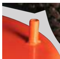
Deck cleaning pipe for connecting water hose
