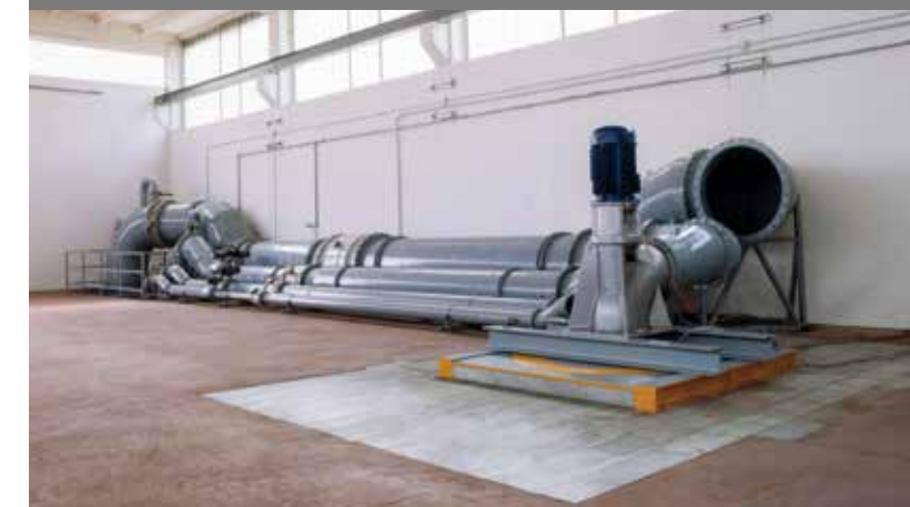
Sala prove | Testing Room
